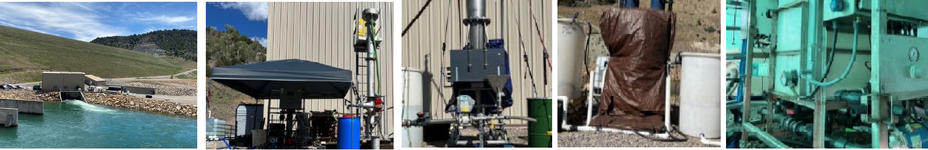
Pilot Site at Ridgway Reservoir Dam Veolia PSR Pilot Study WesTech PSR Pilot System WesTech Granular Media Filter Pilot System MEMCOR UF Pilot System
