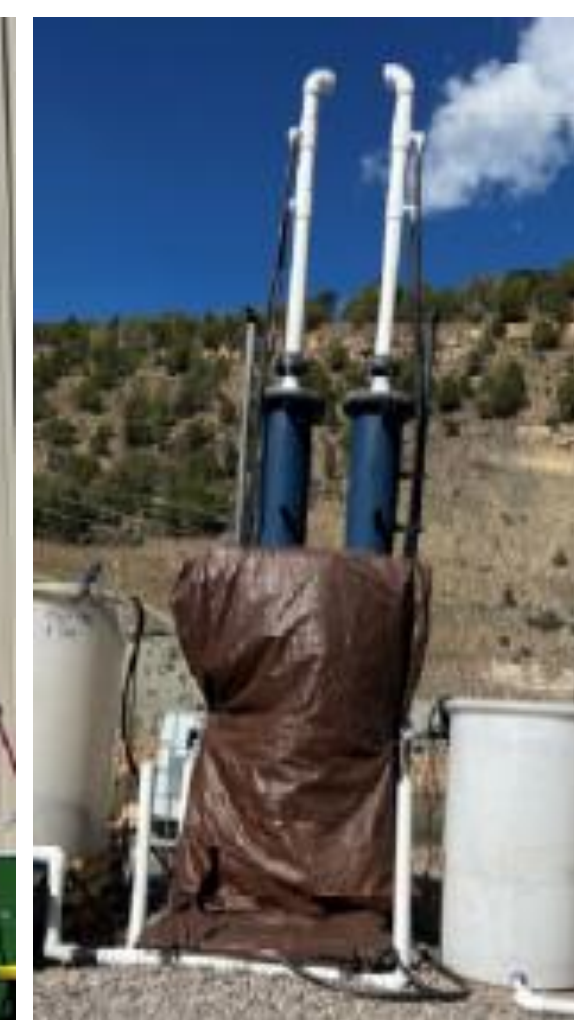
WesTech Granular Media Filter Pilot System
